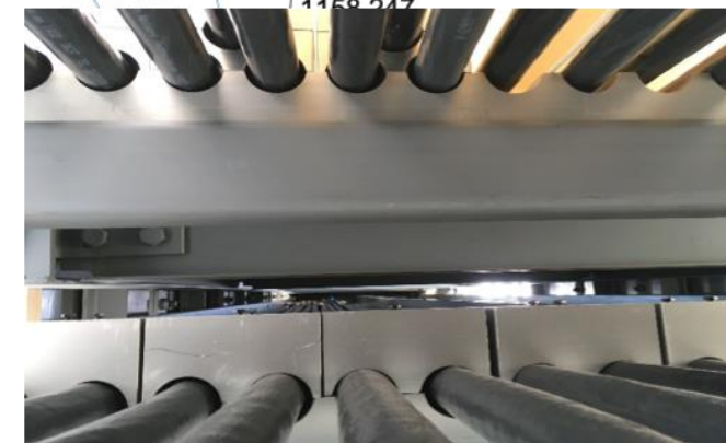
Cables entering the ICL
