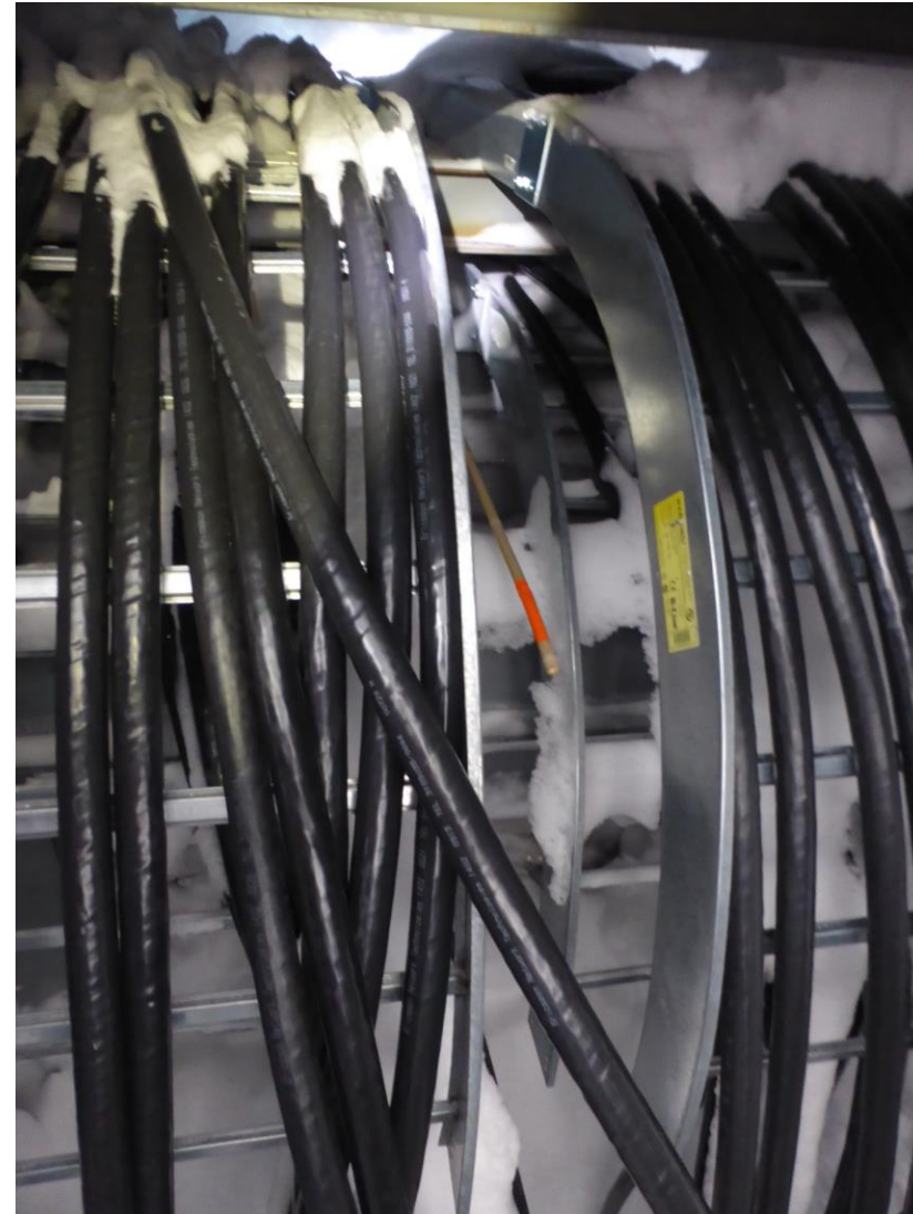
culvert entry cable trays
