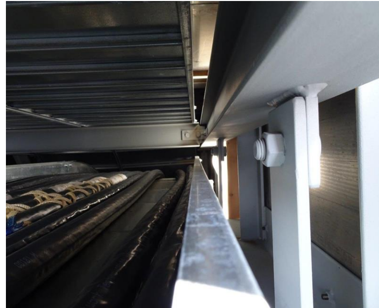
cable bridge lower level
